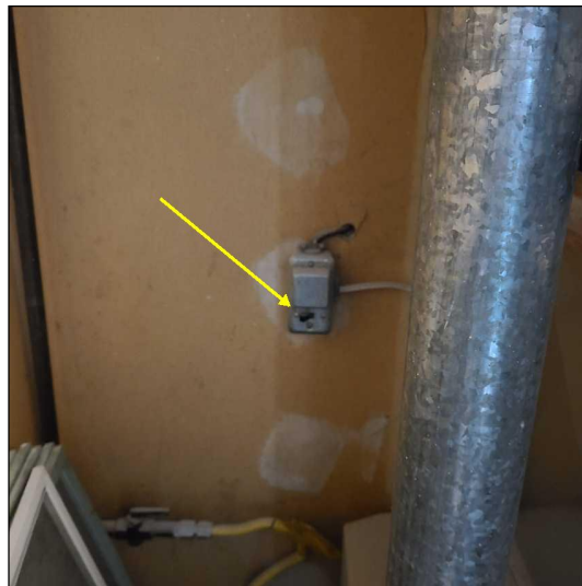
Heater electrical shut off switch
