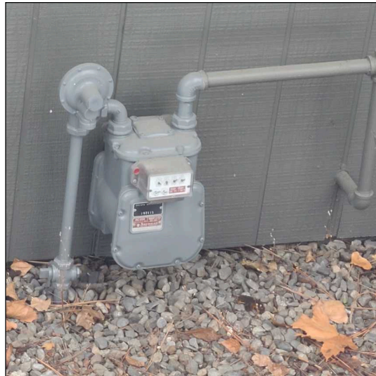
Natural gas meter at rear of home
