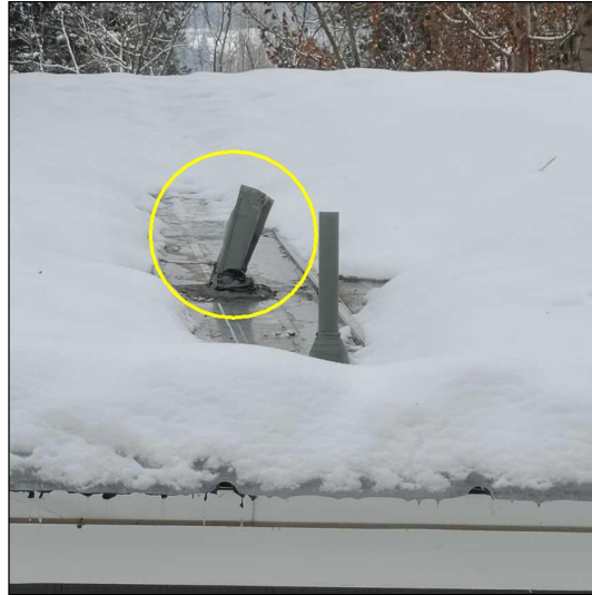
Bent roof vent. Unknown origin.
