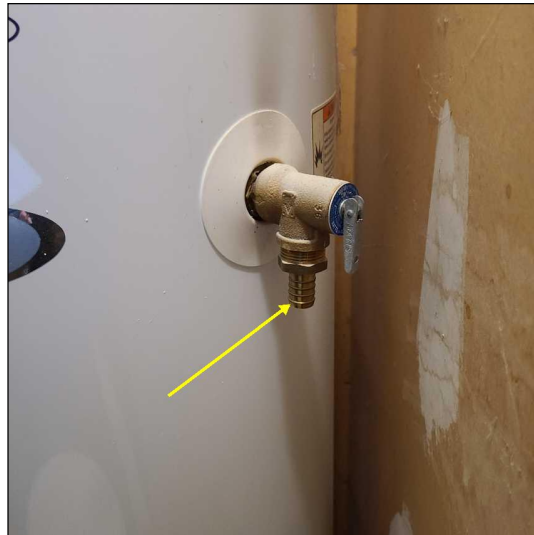
TPR valve not plumbed.
