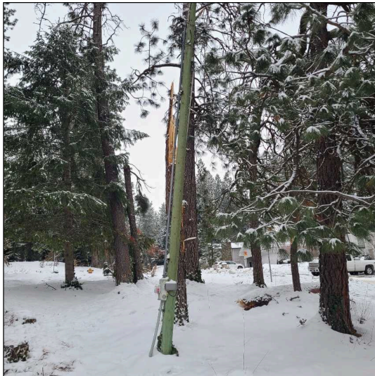
Leaning electric pole.
