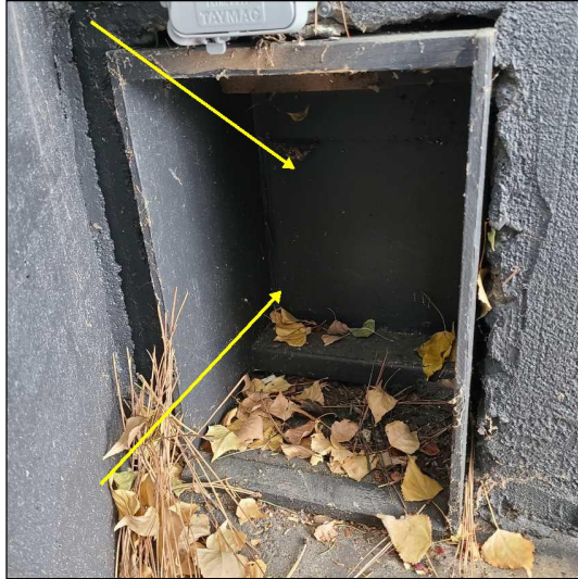
Opening in west wall exposing interior drywall to elements.
