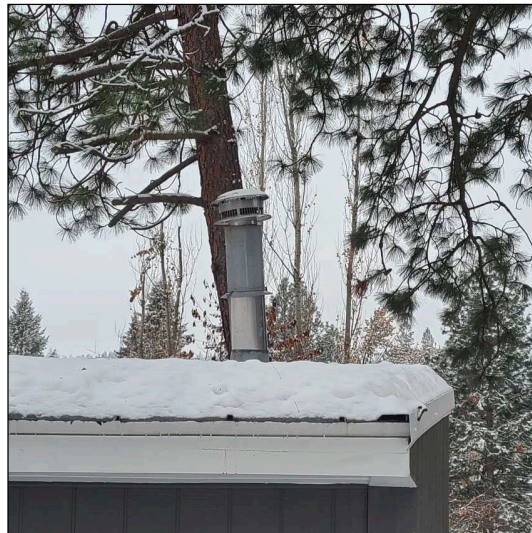
Chimney has no source within home.
