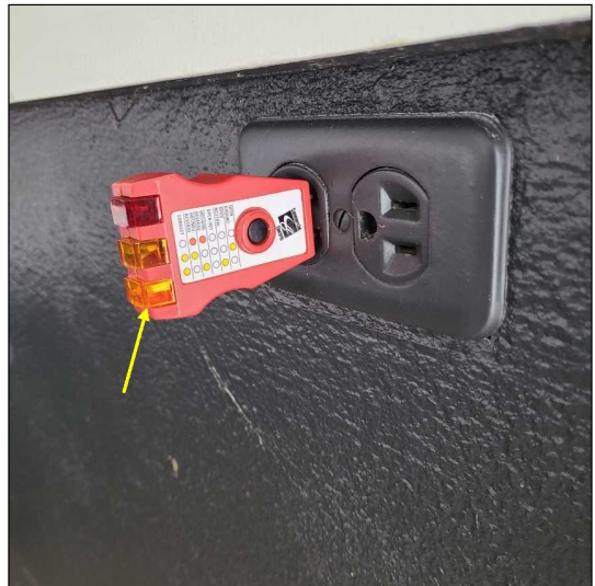
Neutral fault on outlet outside west wall
