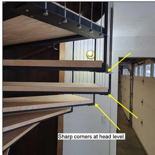
Low stair treads. SAFETY ITEM
