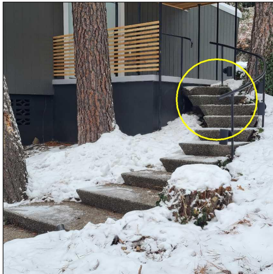
Front steps railing not to end of steps.
