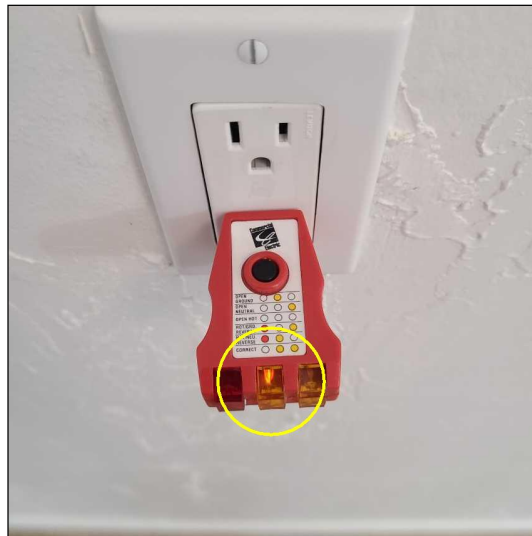
Open Ground on outlet in basement living area.
