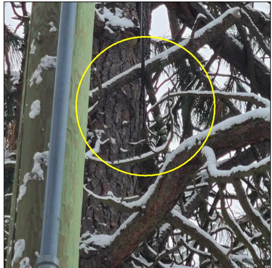
Power lines in contact with tree
