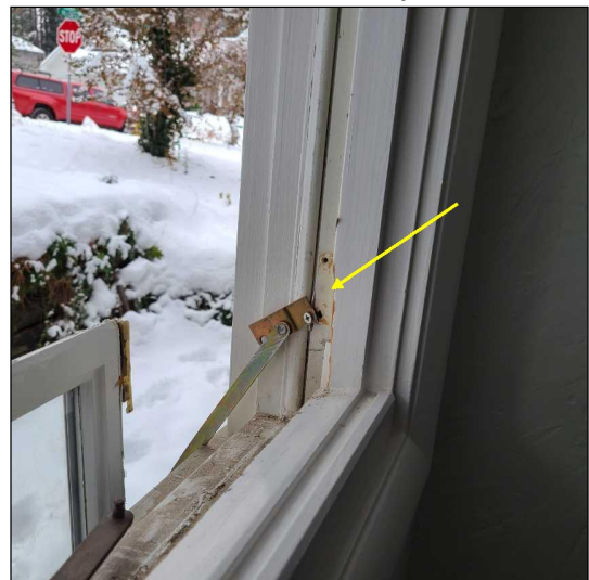
Window hardware damaged.
